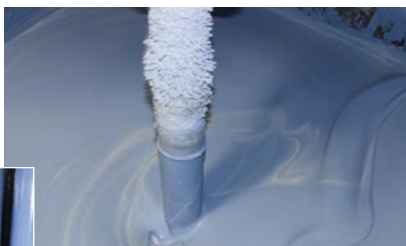
▲ All Vitraglas® components are mixed to create liquid slurry prior to spray application
